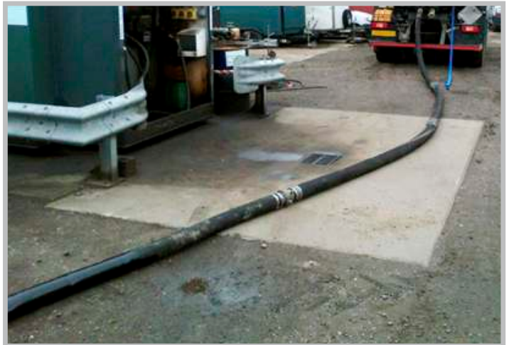
Figure 1. Four hose sections joined together in a vacuum tanker operation with an OhmGuard ® hose tester testing the first hose section (blue cable).
